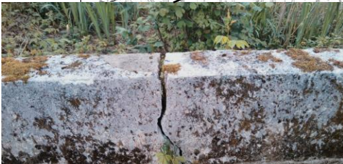
Fissuration muret béton
